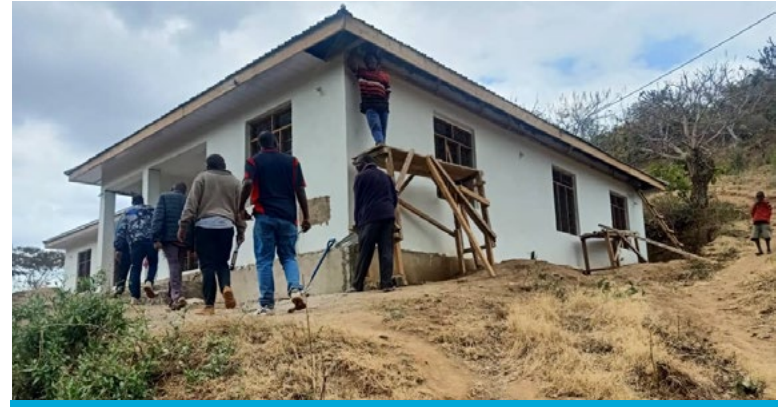
Experts/engineers attending to a Governor's residence house construction, one of the Tanga Regional Secretariat projects
