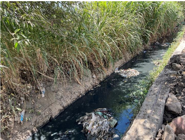
Figure 6 Clogged drainage system.
