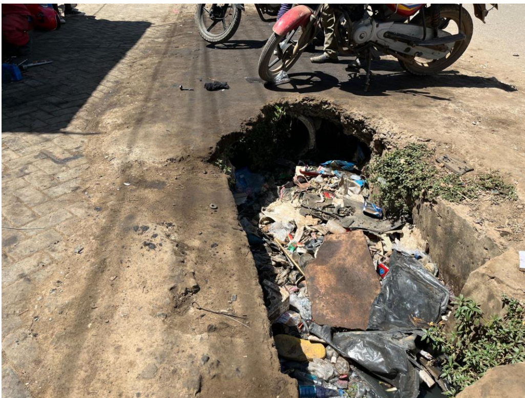
Figure 6 Garbage disposed off in drainage.
